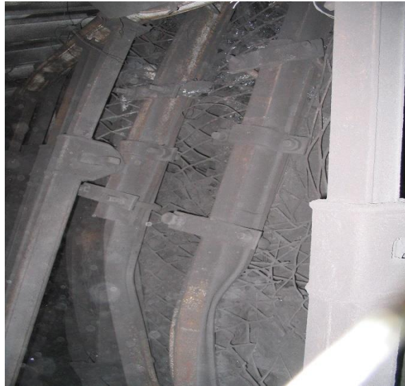
deformation of arch support pillars
