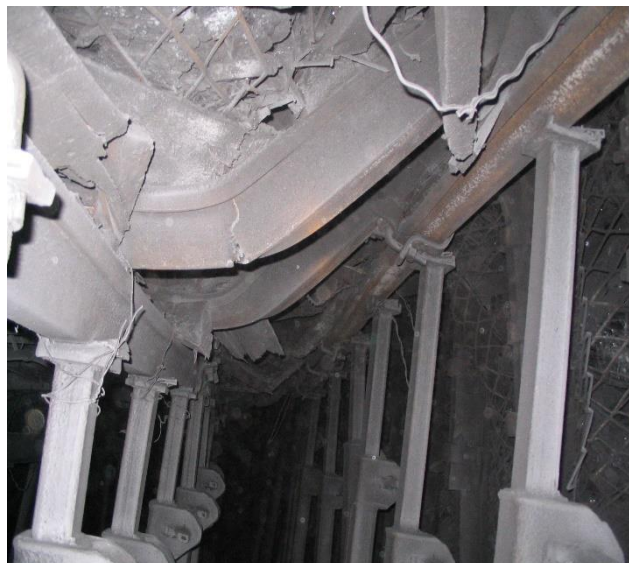
deformation of the top
